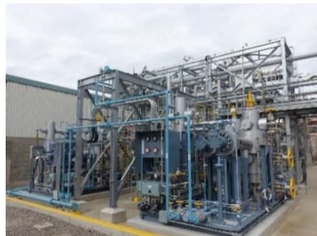
2 Pilot facilities manufacturing at high efficiency methanol from CO 2
