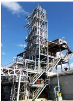
4 Chemical recycling demonstration facility
